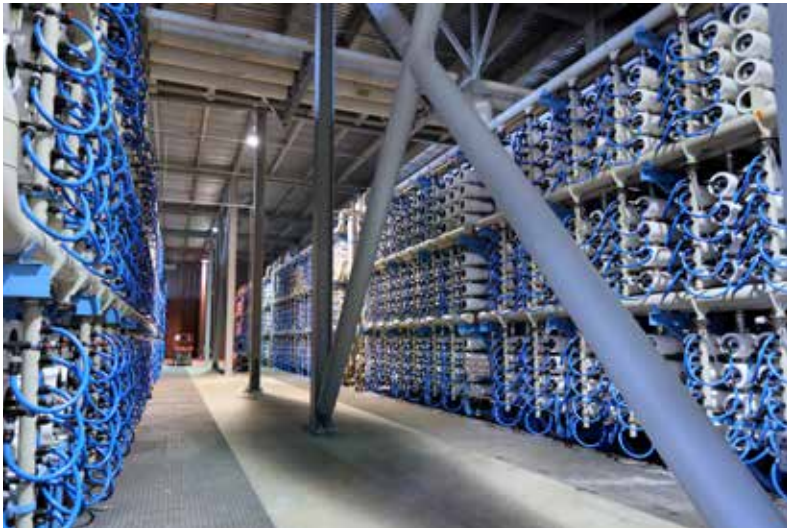
The heart of the Carlsbad Desalination Plant is a reverse-osmosis system designed by IDE Technologies.
