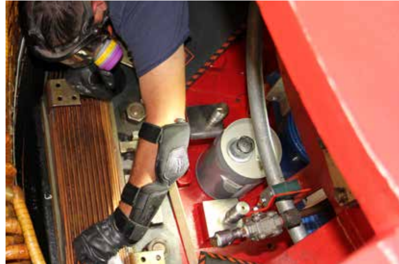
An Operations and Maintenance technician attends to repairs at the Lake Hodges Pump Station.
